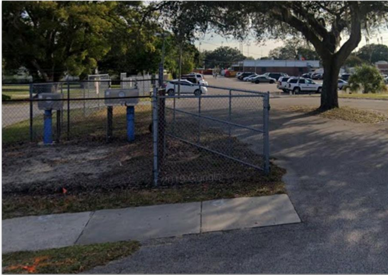
Monitoring Wells at Chamberlain High School
